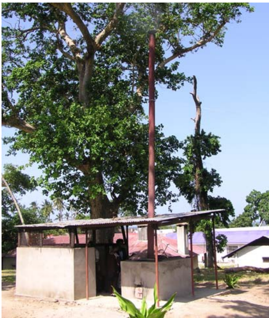
The incinerator at BDH before its breakdown
