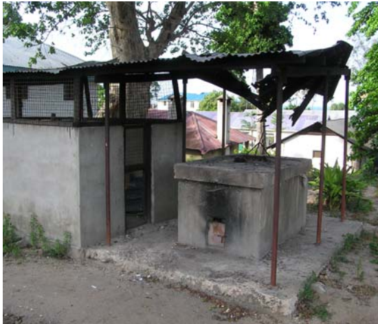
Incinerator with stack and roof burnt out
